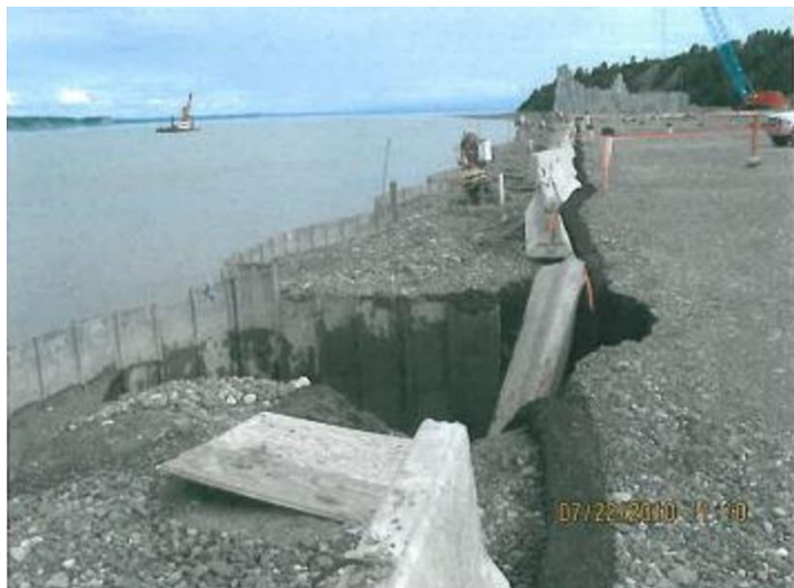
Figure 11. Subsidence of Impounded Materials at the Face Wall (Bulkhead) Illustrating Material Loss Through the Face Sheet Interlocks
