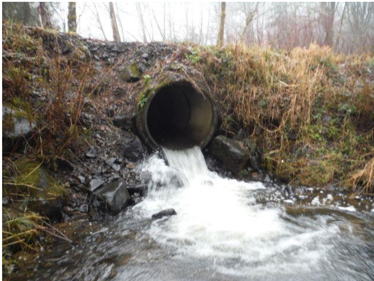
Photo: Fish passage barrier culvert. Credit: Washington Department of Fish and Wildlife.
